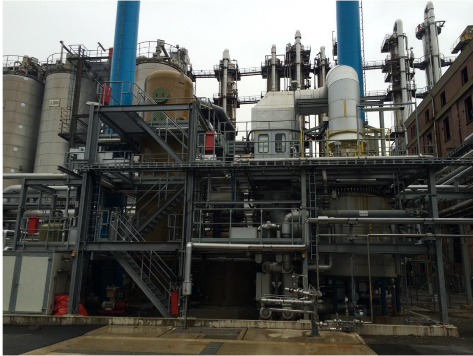
The gas scrubber
